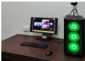
Shahmim Irshad - High Performance Computing Facility
