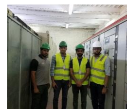
Energy Audit of Electric Panels
