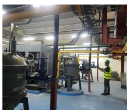
Energy Audit of Compressors
