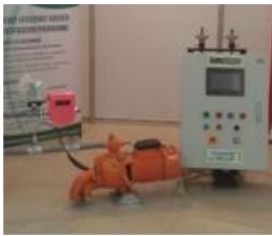
Manel Control Panel view
