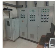
CONTROL PANEL FOR AC TESTING LAB
