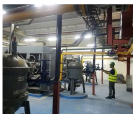
Energy Audit of Compressors
